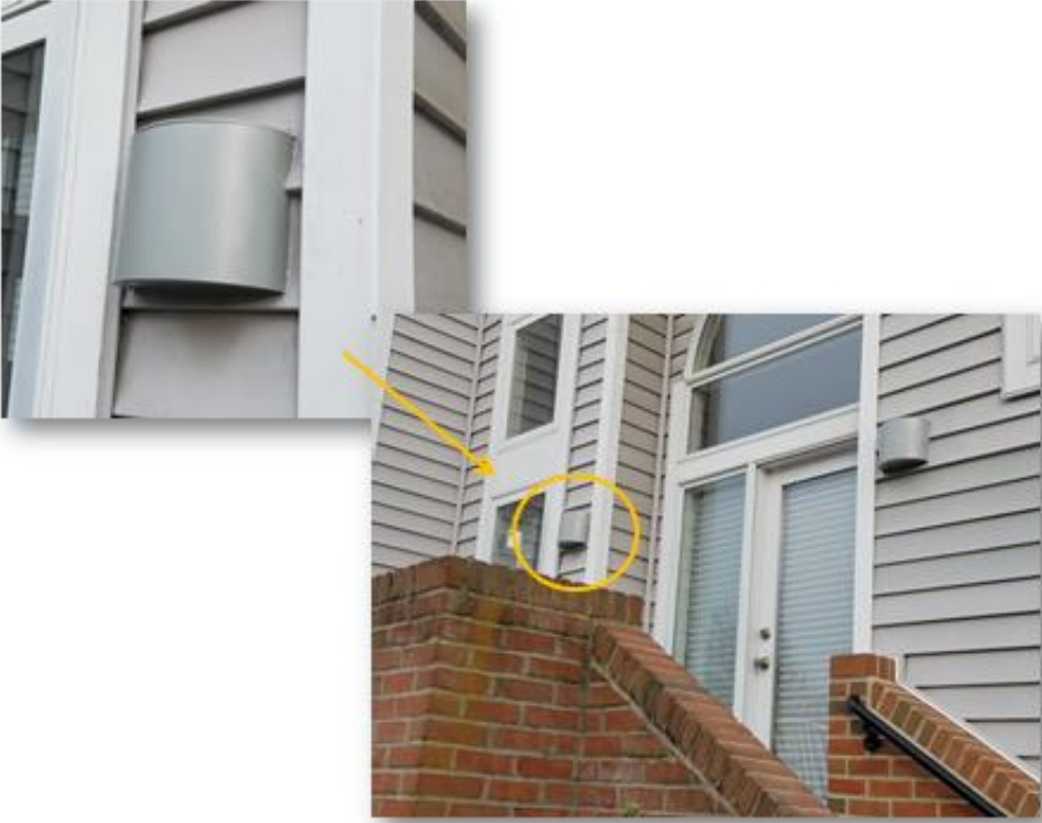
Hinkley 1667TT front entrance lighting at 405 Martingale Lane
